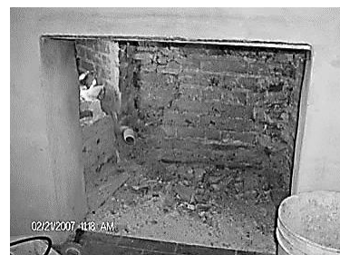
Badly Deteriorated Firebox
