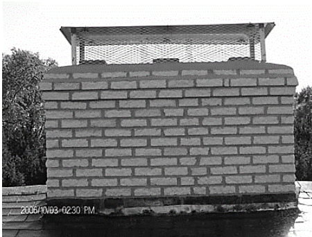
Metal Cap on Clay Liner Chimney Top
