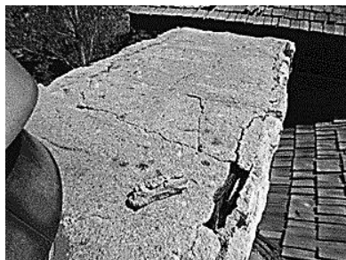
Damaged Chimney Cap
